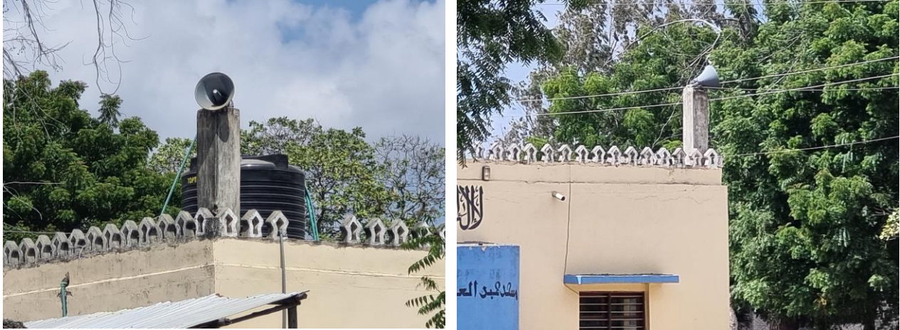
Plate 4-3: One of the Public Address systems noted in the area
