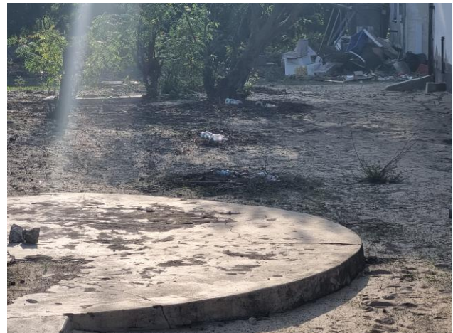
Plate 4-14: One of the Septic Tanks serving the Fisheries office at Amu Island
