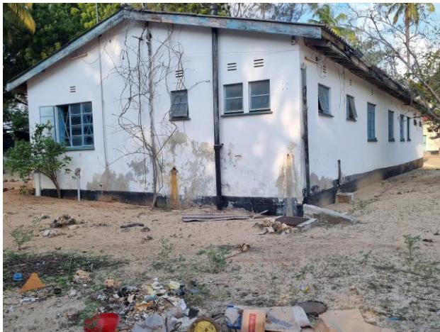
Plate 4-13: Fisheries office connected to water closet toilet at Amu Island
