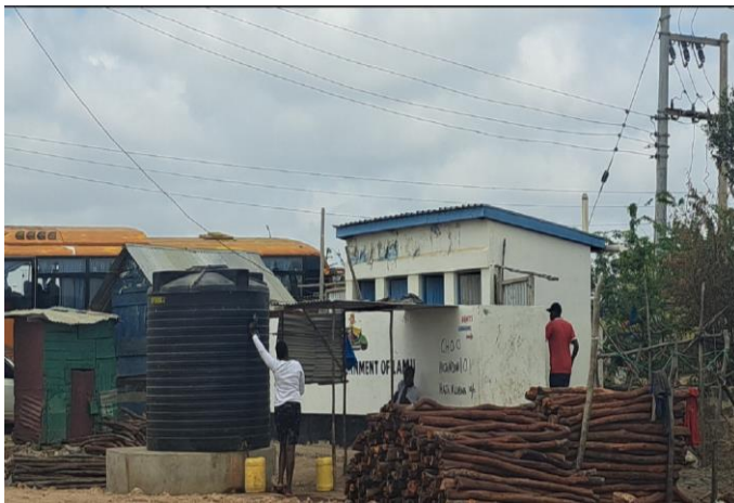
Plate 4-15: Storage tank at the Public Toilet supplied by a water bowser sourcing water from Hindi area
