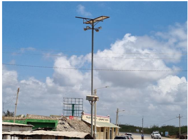
Plate 4-23: Solarised Street Lights at Mokowe Landing site area
