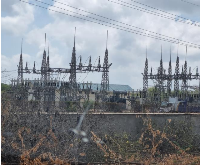
Plate 4-20: Power Supply Sub-station noted at Mokowe Area
