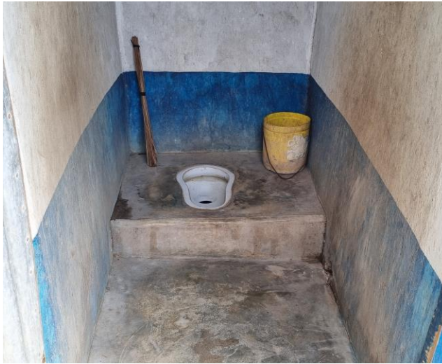
Plate 4-16: Toilet Connected to A soak pit
